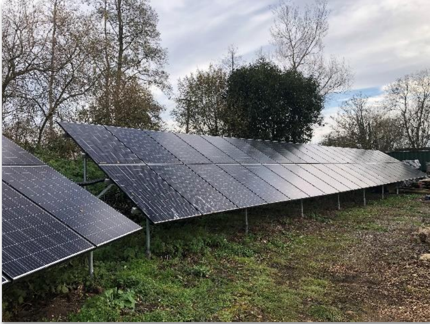
Figure 8: Solar photovoltaic panels situated in working yard, adjacent to compost heaps.
