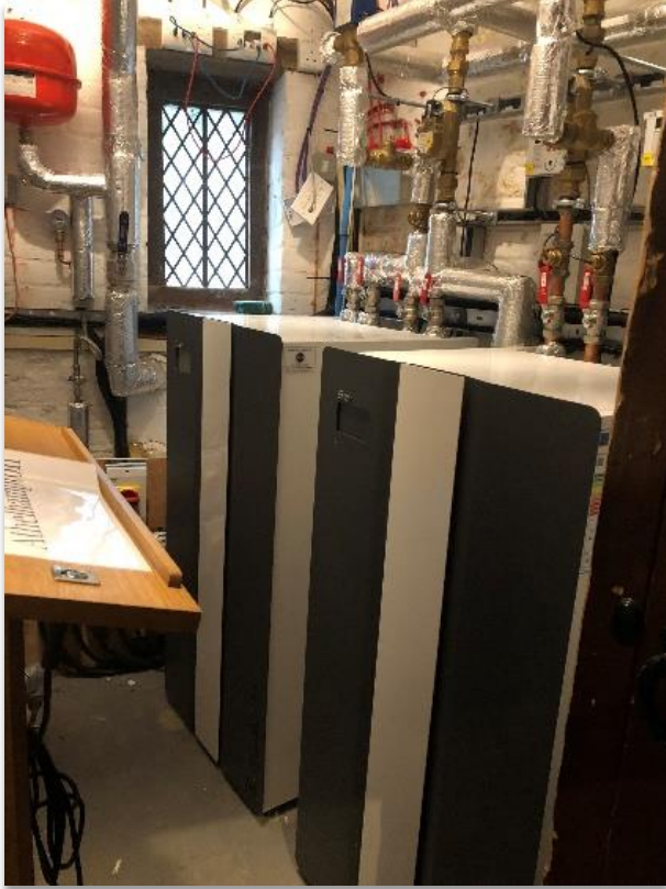
Figure 6: Ground source heat pump equipment sited in a room at the back of the building.
