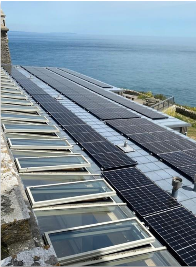
Figure 4: Installed solar panels
