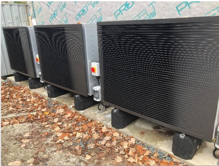
Figure 9: Air source heat pumps at the side of a modern building.
